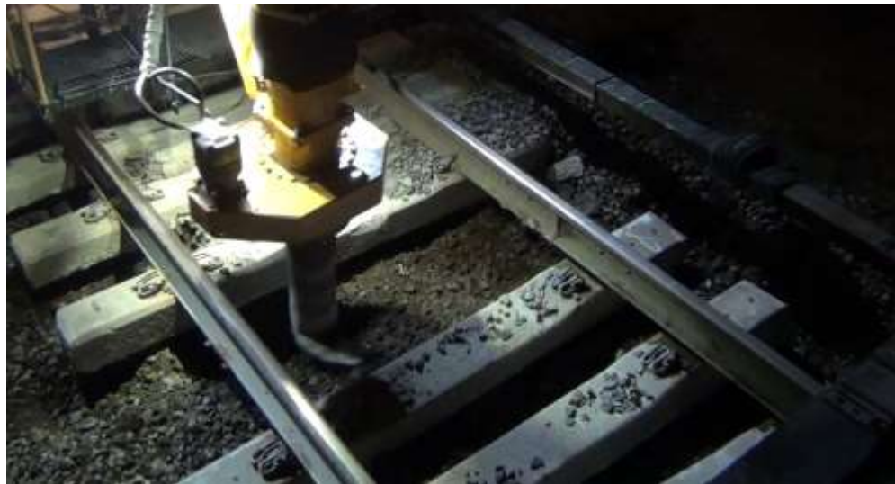
Railvac Undercutting-Notice Third Rail and Dropped Ties
